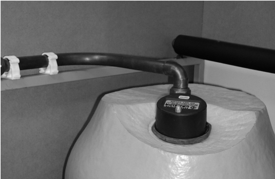
fig 138: outlet pipe from top of cylinder
