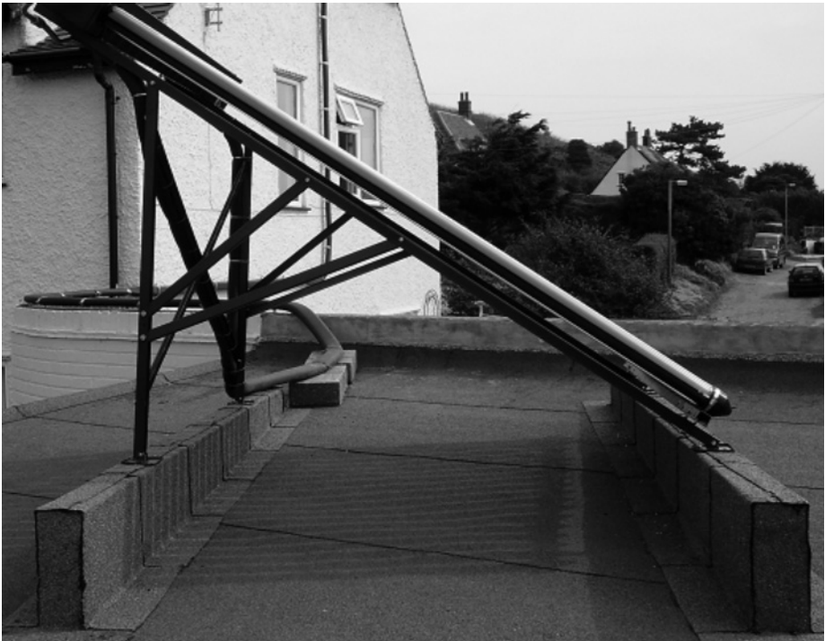
fig 122: roof collector mounted on weather-resistant timber bearers
