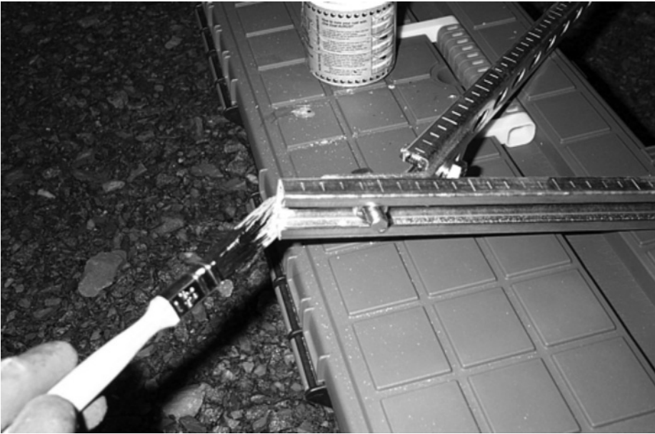
fig 120: protect exposed ends against corrosion
