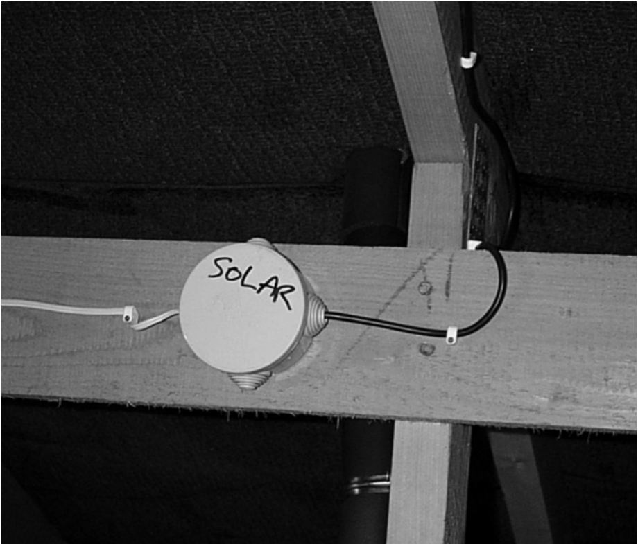
fig 148: clearly marked junction box
