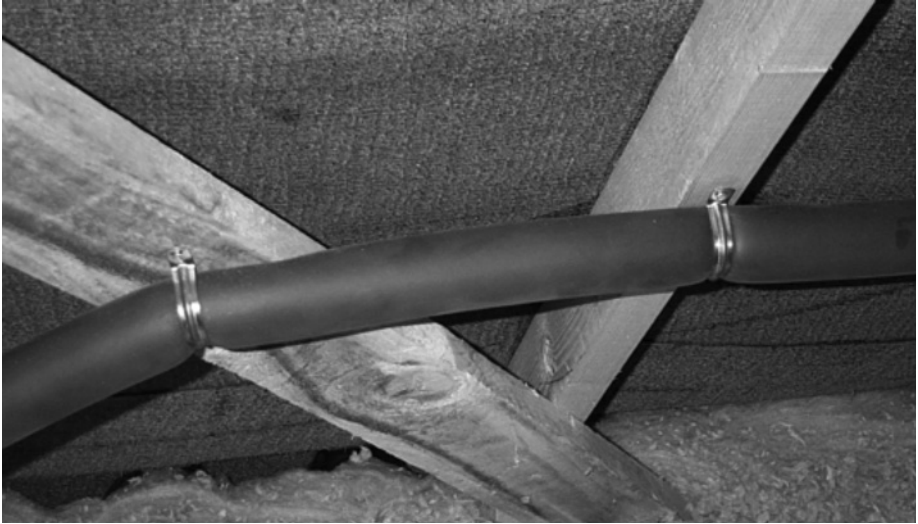
fig 97: an insulated pipe in situ
