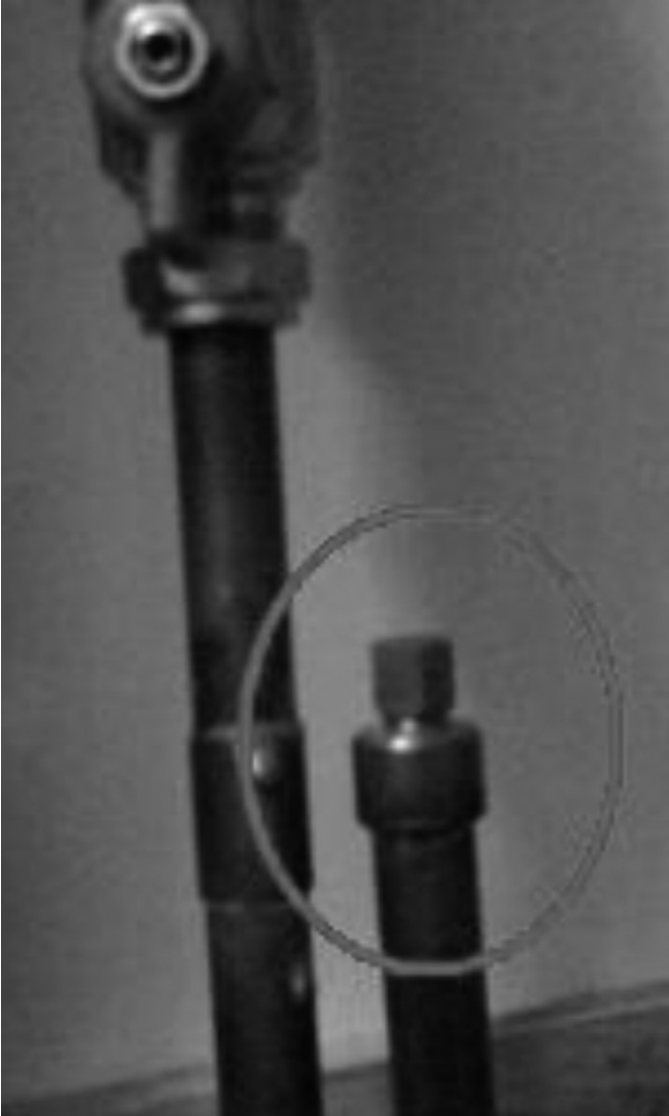
fig 73: air release cap (circled)
