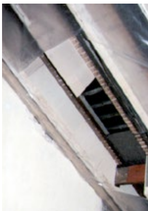
Figure 6.8 Recess for rooflight in 300 mm deep extension rafters with air/vapour barrier and plasterboard. Picture: Gil Schalom
