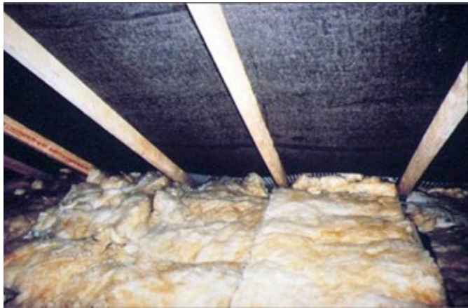
Figure 6.1 Mineral wool quilt insulation in a loft
