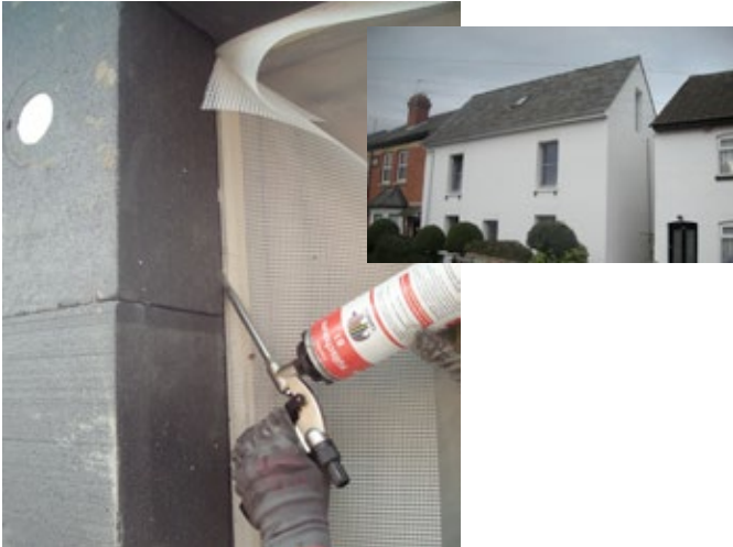
Figure 5.8 The gap between 250 mm thick grey polystyrene insulation and a window frame being sealed with expanding foam prior to rendering at Grove Cottage, Hereford. Pictures: Simmonds Mills Architects
