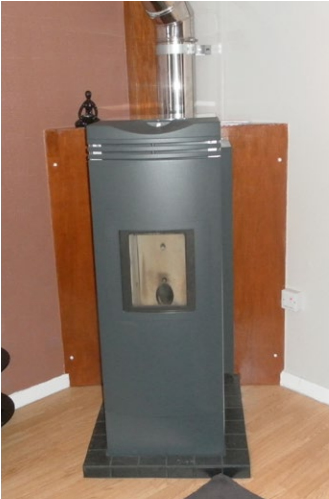
Baxi Bioflo boiler installed
