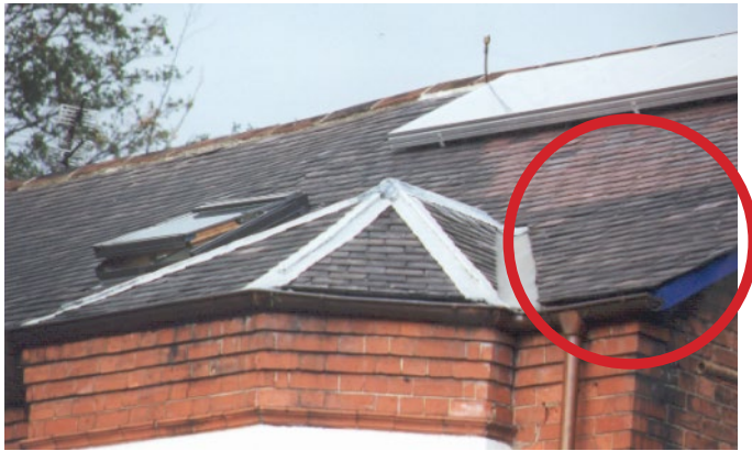
Figure 3.1 Extended roof verge to accommodate future external wall insulation. Picture courtesy of Gil Schalom
