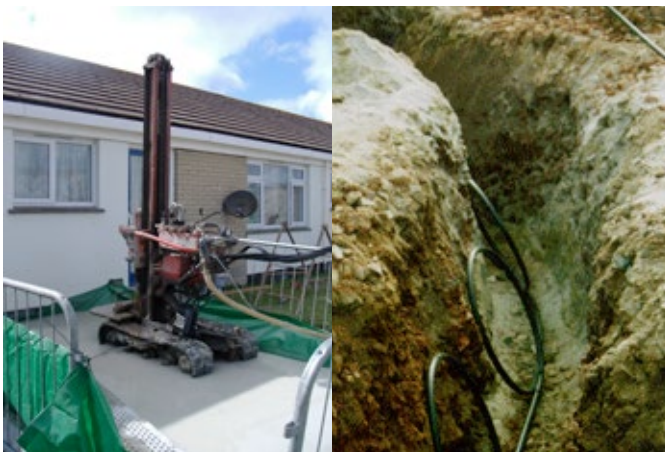
Figure 10.3 Borehole drilling rig and ground loops, for ground source heat pumps. Pictures courtesy of DCH
