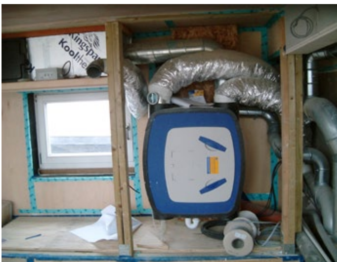
Figure 9.7 Heat recovery ventilation in a refurbishment project in Hackney (note the conglomeration of ducts and also the extensive use of sealing tape). Picture: John Willoughby
