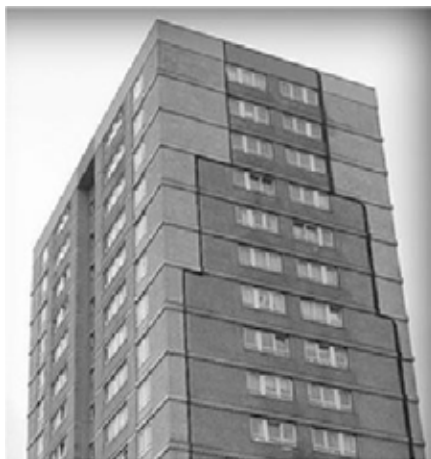
Figure 5.3 A high-rise block in Edinburgh insulated with proprietary polyurethane cavity wall insulation. Picture: Isothane
