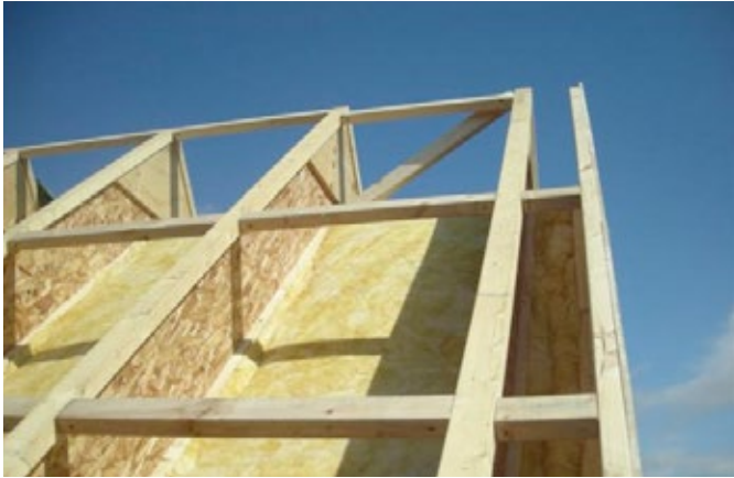
Figure 6.3 400 mm deep engineered timber 'I beams' with the first layer of roof insulation over the existing roof structure. Picture: Simmonds Mills Architects
