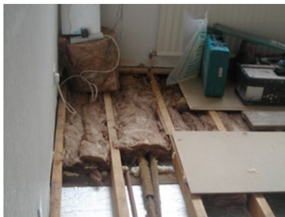
Figure 4.2b Insulating below the joists keeps timbers and pipes warm Picture: John Willoughby
