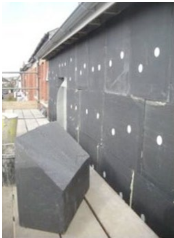
Figure 6.4 The 250 mm thick external wall insulation, with a block shaped to fit at the eaves. Picture: Simmonds Mills Architects
