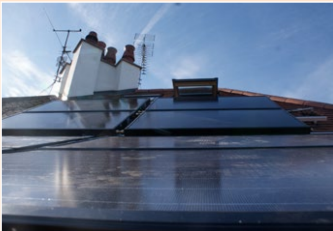
Solar system and passive ventilation chimney stack
