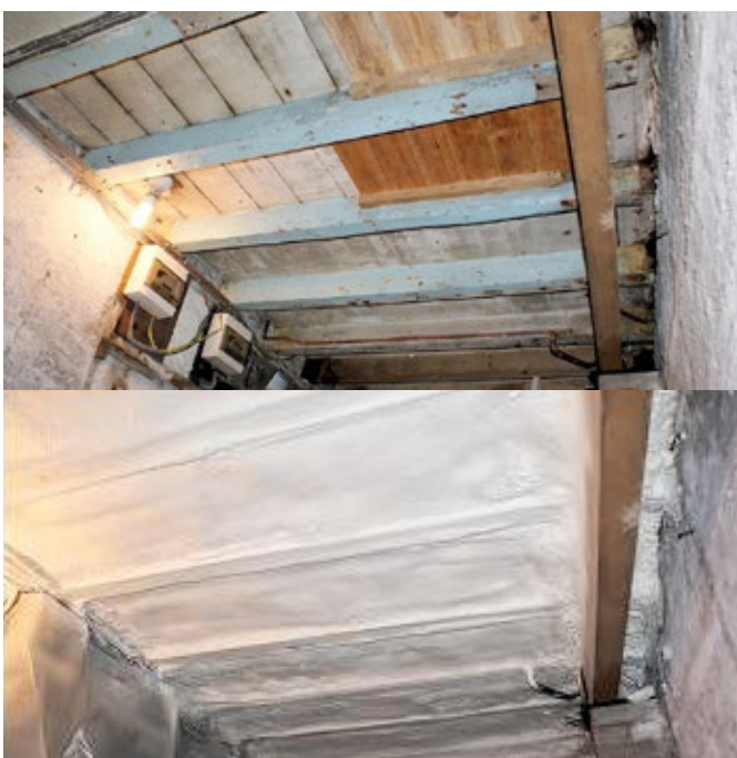
Figure 4.5 The floor seen from the cellar; before and after the installation of spray-applied polyurethane insulation. Pictures: Isothane
