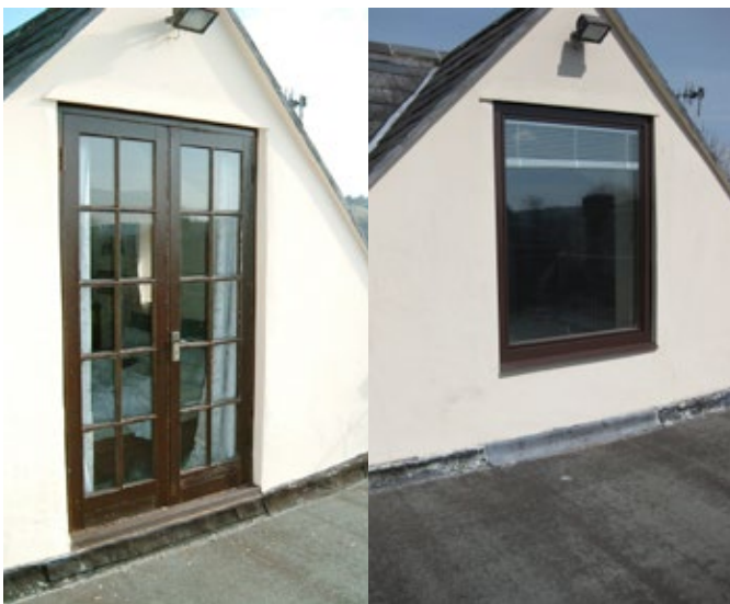
Figure 3.2 Door replaced by a window to accommodate future flat roof insulation. Pictures: John Willoughby
