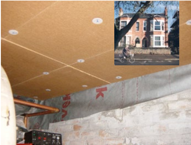
Figure 4.3 Insulating a suspended floor from beneath, at the Nottingham EcoHome. Picture courtesy of Gil Schalom
