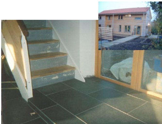
Figure 4.9 A landing built at the bottom of stairs to even out the risers. Pictures: Tony Cleford
