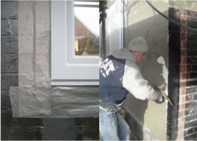
Figure 8.6 Windows taped to walls before they were rendered and covered with 250 mm of insulation. Pictures: Simmonds Mills Architects
