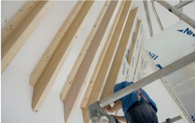
Figure 6.6 Z rafters were set out using a jig to ensure the spacings matched the rigid insulation board. Picture: Ray Exton
