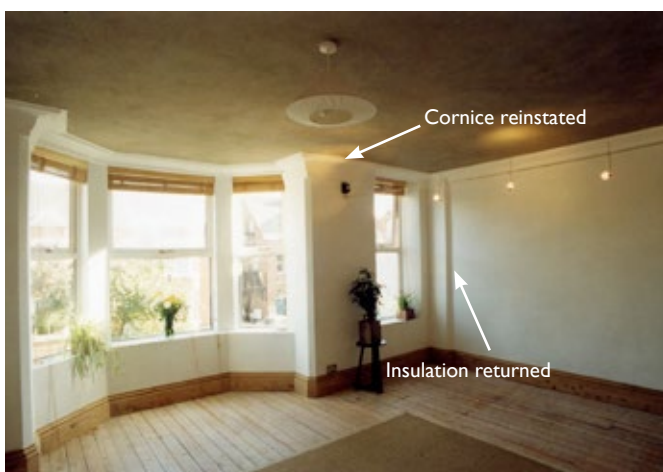
Figure 5.17 Internal insulation at the Nottingham EcoHome – note the reinstated coving and the insulation returned along the party wall. Picture: Gil Schalom
