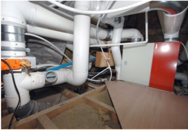
Ventilation ducting in loft
