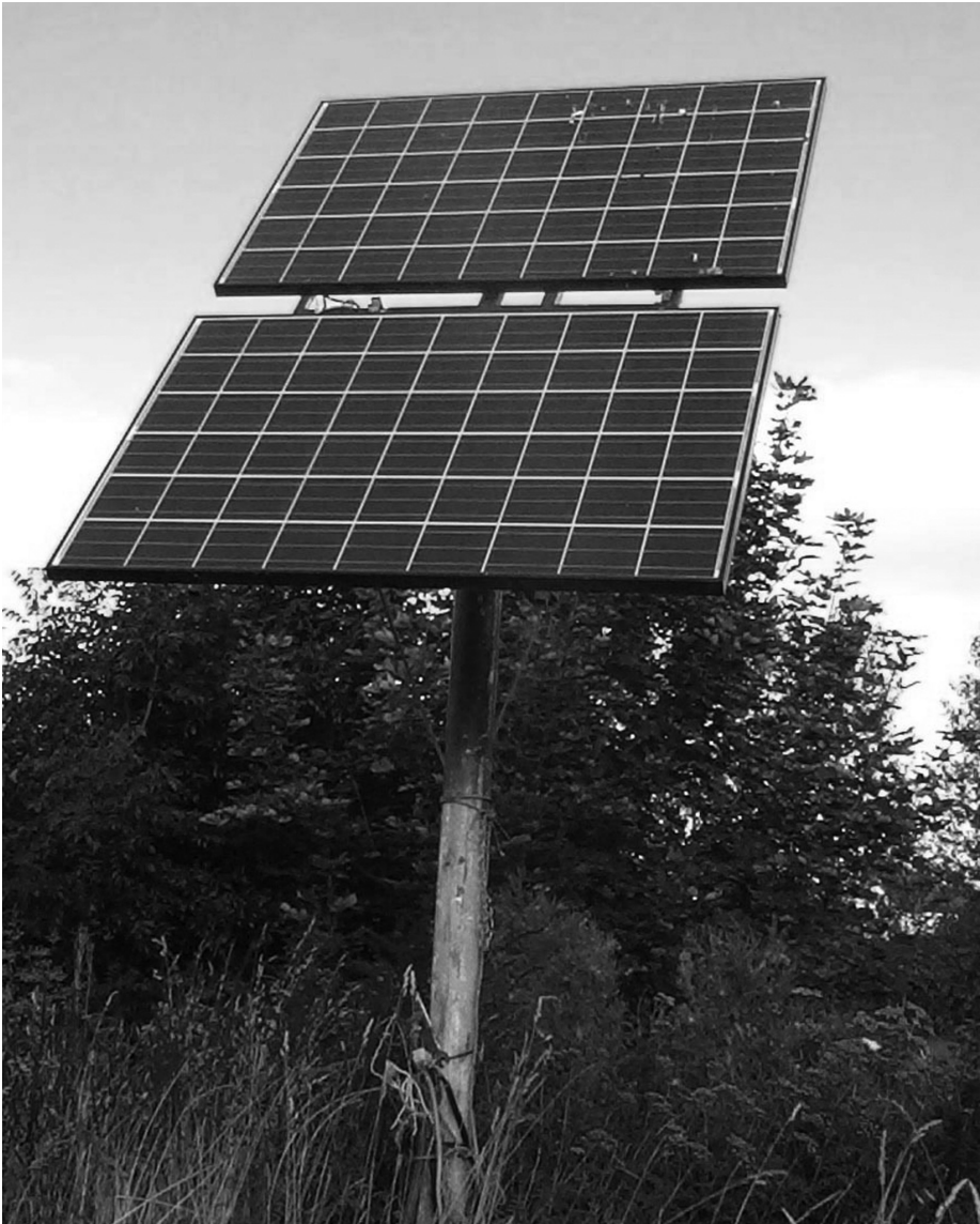
fig 26: pole mounted solar array
