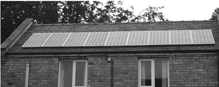
fig 28: roof-mounted solar array
