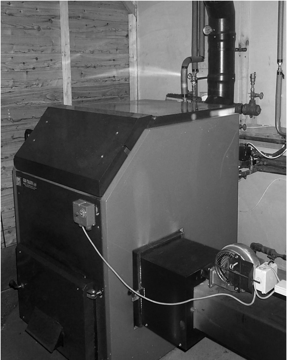
fig 33: 70Kw Alcon biomass boiler
