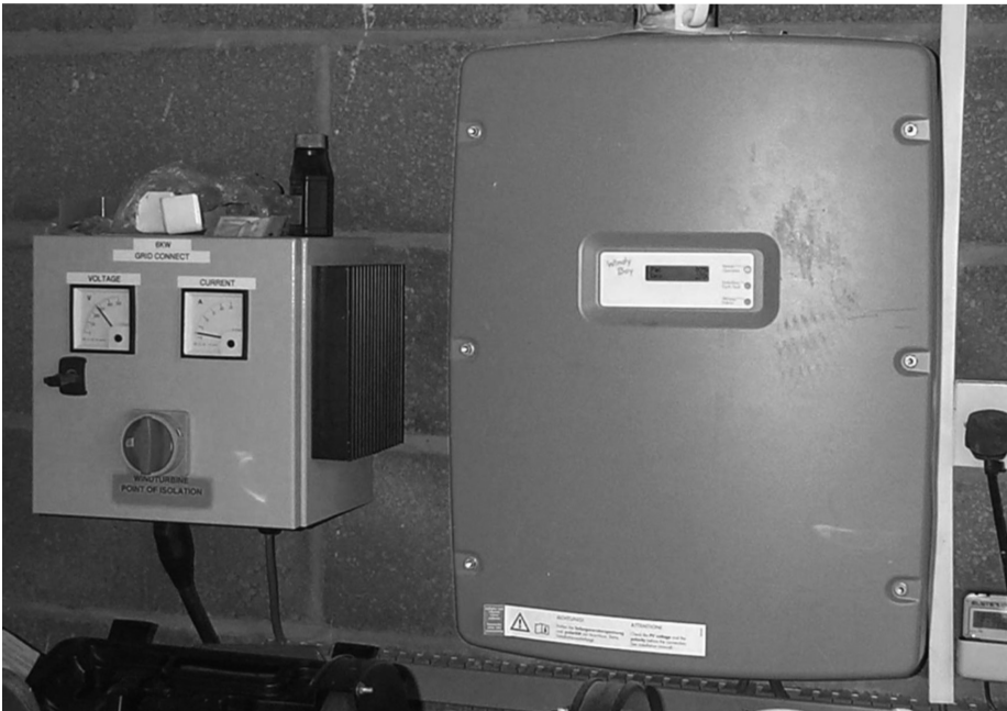
fig 51: 6 kilowatt grid-tie inverter (right) and turbine controller (left)
