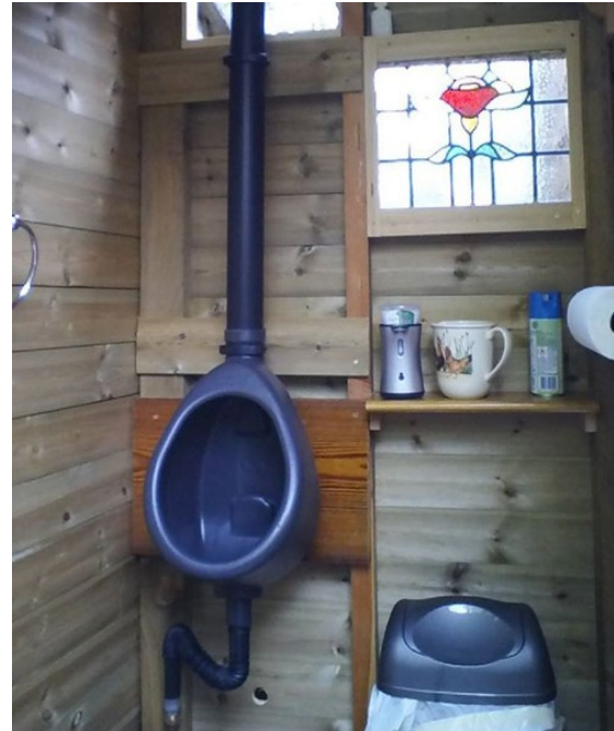
Shed installation of the vented Biolan Urinal in Cornwall. No trap – the urine is just led away to the ground or to a straw-bale / sawdust pile to create compost. Good for allotments / gardens.
