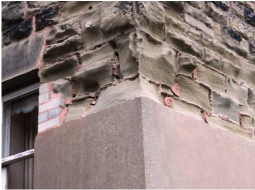
Damage to a stone wall due to the inappropriate use of cement mortar & render.
