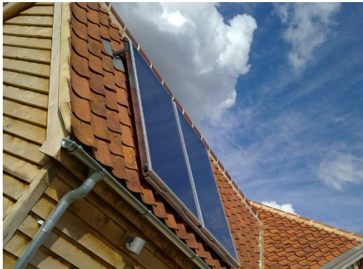
2 flat-plate panels on a domestic roof; they're thicker than solar electric panels, but only protrude about 10cm from the roof.
