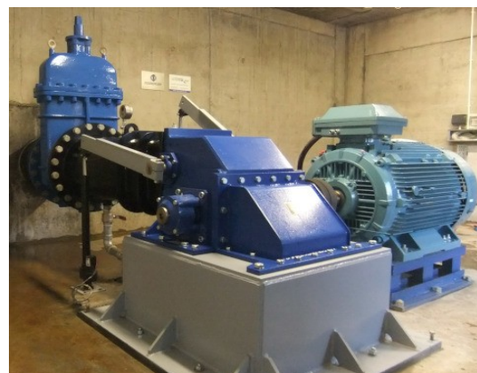
Micro-hydro turbine in operation.
