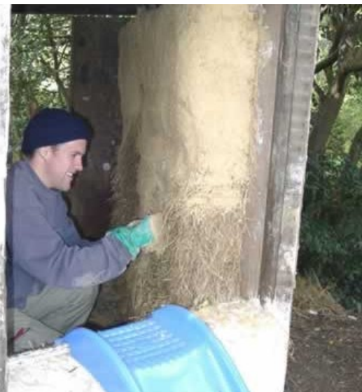
Lime rendering a straw-bale play-house: one part lime putty is mixed with 3 parts sharp sand. The walls are sprayed with water first; apply two coats, and allow each to dry slowly by covering with wet sacking.
