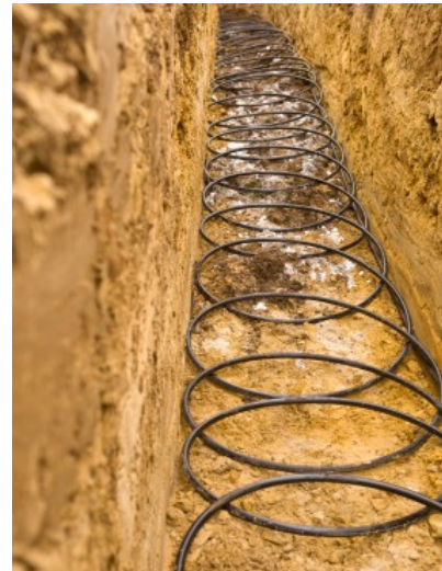
Loopy collector pipe for a ground-source heat pump being laid in a trench.
