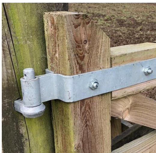
Detail of gate hinge. There's a vertical pin that fits through an eye on the gate bolt / bracket – the gate is lifted on, and is kept in place by gravity.
