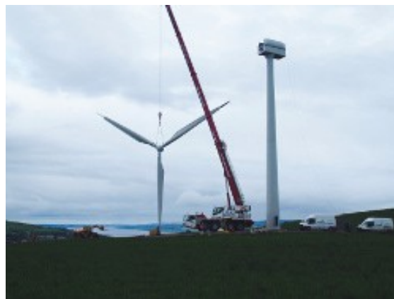
Blades being attached to Scotland's first 100% co-operatively-owned wind turbine, owned by Dingwall Wind Co-op.
