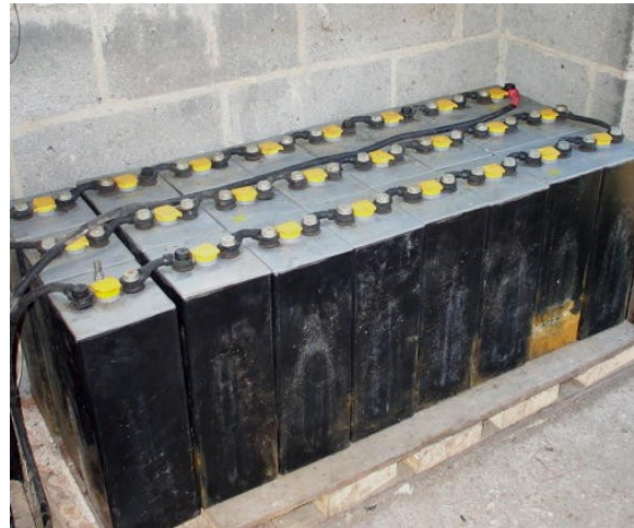
A collection of 600 amp-hour, 2-volt cells wired in series (a 48-volt battery pack); 600 \times 48 = 29\text{kWh} , and so the available power is 50% of this (you should never discharge a battery to less than 50% of its capacity), or 14.5kWh.
