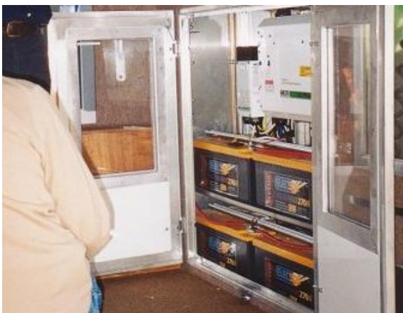
4 leisure batteries and an inverter on a vehicle with 12 x 80-watt PV panels on the roof, plus a 350-watt wind turbine.
