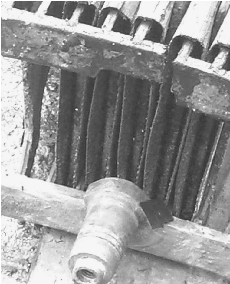
fig 42: positive bar corrosion
