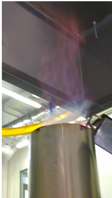
Fig. 22: gasifier flare stack during start-up showing transition to blue flame
