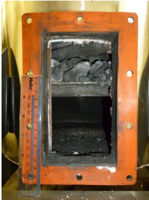
Fig. 11: view inside the gasifier reactor showing the charcoal at the base of the reduction zone supported on the ash grate. The ash grate has recently been cleaned out in this photograph.
