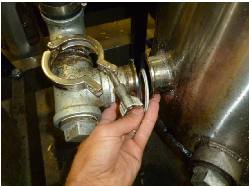
Fig. 28: tar visible on gasifier steel components
