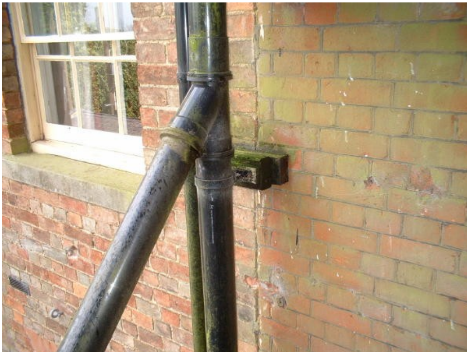
Because of internal plaster, the vent pipe is closer to the wall inside than it is outside. Vent pipe comes with special brackets, and to make up the extra distance between the pipe and the wall, the bracket is fixed to a block of wood.
