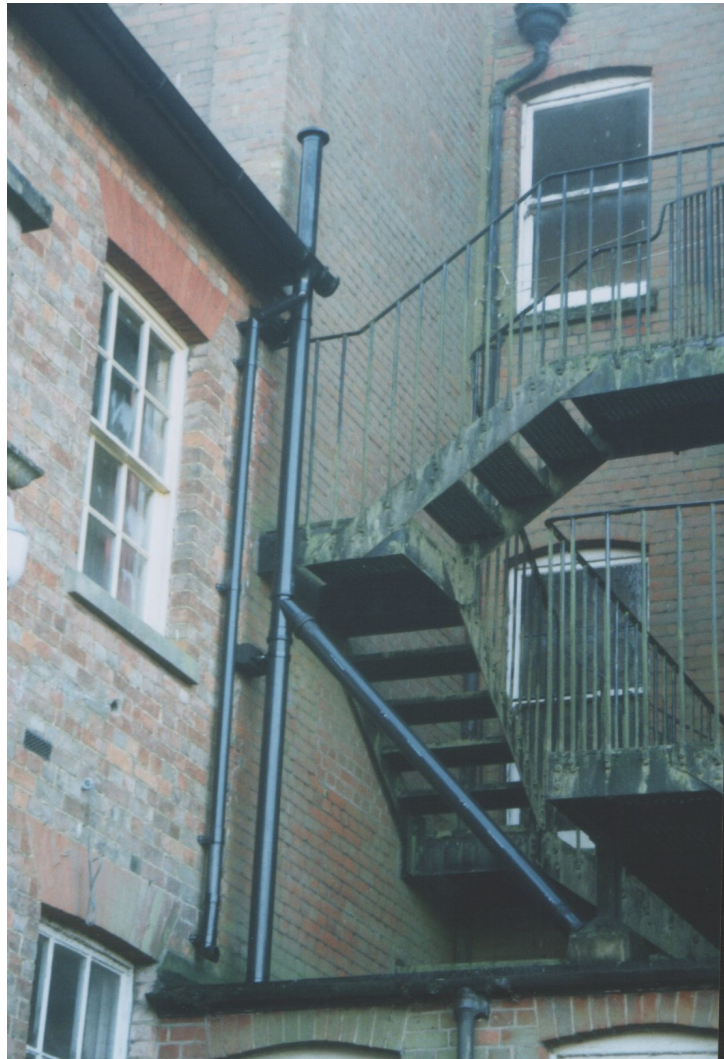
The vent pipe from the left-hand chamber rises vertically from the chamber, through the roof and above the gutter line. The vent from the right-hand chamber comes through the roof and meets a 45° bend, then rises at 45° until it meets the other vent pipe at a 45° tee. These fittings can be bought at good plumbers' merchants.
