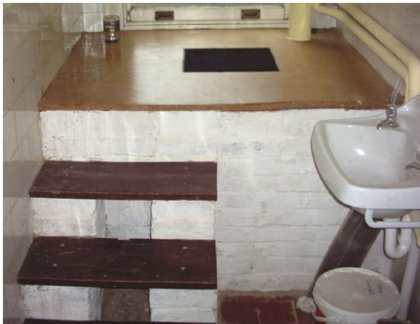
This picture shows a chamber with steps, platform with cork tiles, vent, and fly-trap. the bricks have been limewashed. The chamber has a 10cm layer of sawdust, and is ready for the seat to be attached.
