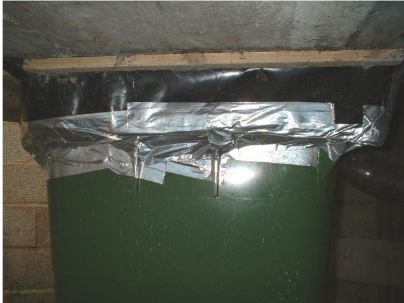
The chute into the wheelie-bin from the room above is secured with 'gaffer' tape to keep out flies.
