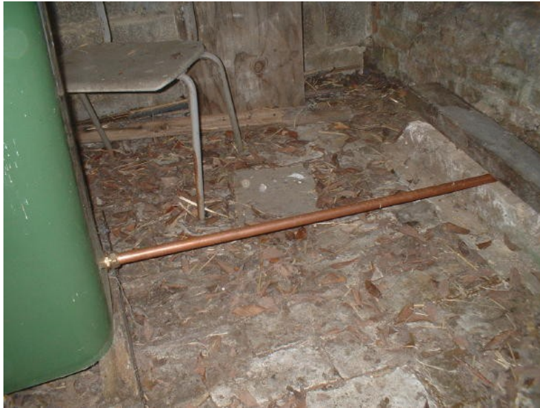
The drain pipe at the bottom of the wheelie bin slopes gently to a sewer drain.
