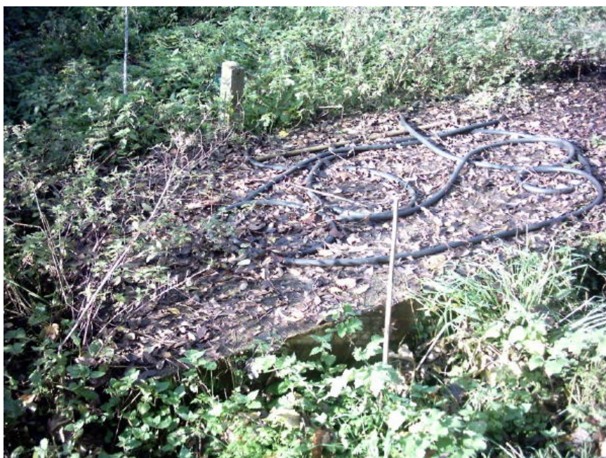
This septic tank (made from concrete, half hidden by vegetation and dead leaves) holds solids and allows liquids to pass through to a rotating-arm sewer; a truck pumps out the contents once a year.
