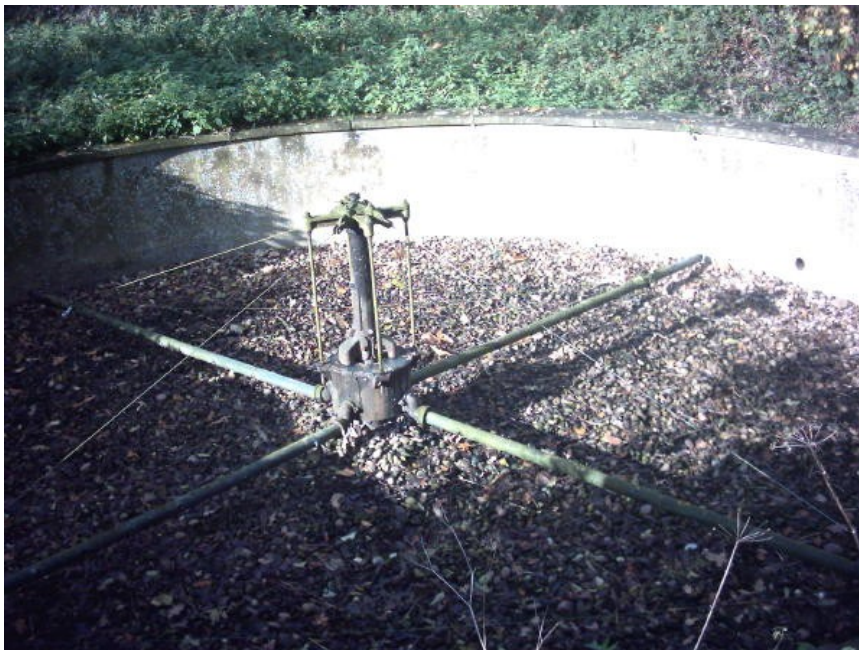
Rotating-arm sewers use no electricity and are very durable; this one was built by the council for Redfield when it was an old peoples' home in the 1950s, and it's still going strong.
