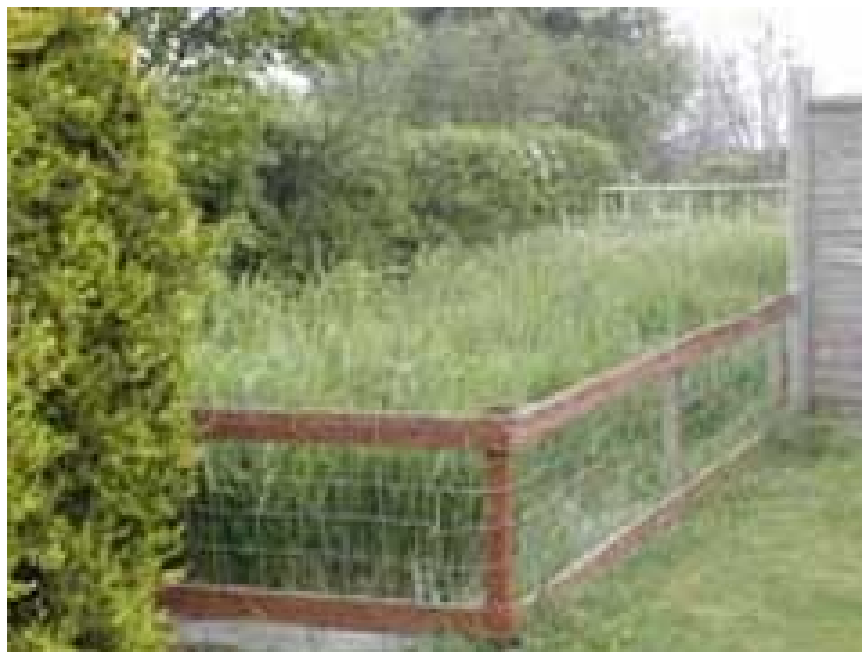
Horizontal-flow reed bed installed by Elemental Solutions at a pub in Worcestershire.
