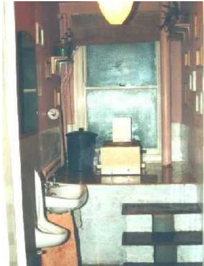
Compost toilet in use: the 'throne' sits on top of the chamber. Note the bucket for sawdust, steps up to platform, vent from chamber through roof and above gutter-line, instructions on wall and waterless urinal in the foreground.
